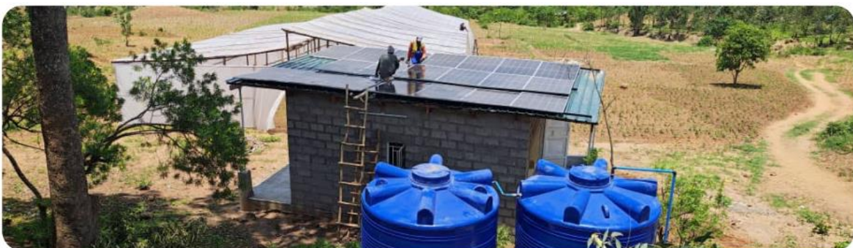
Figure 3-6: A picture showing an example of solar PV energy kiosk that will be used for small scale irrigation and water supply, battery charging, lighting: constructed by RENAMA in Thyolo District
